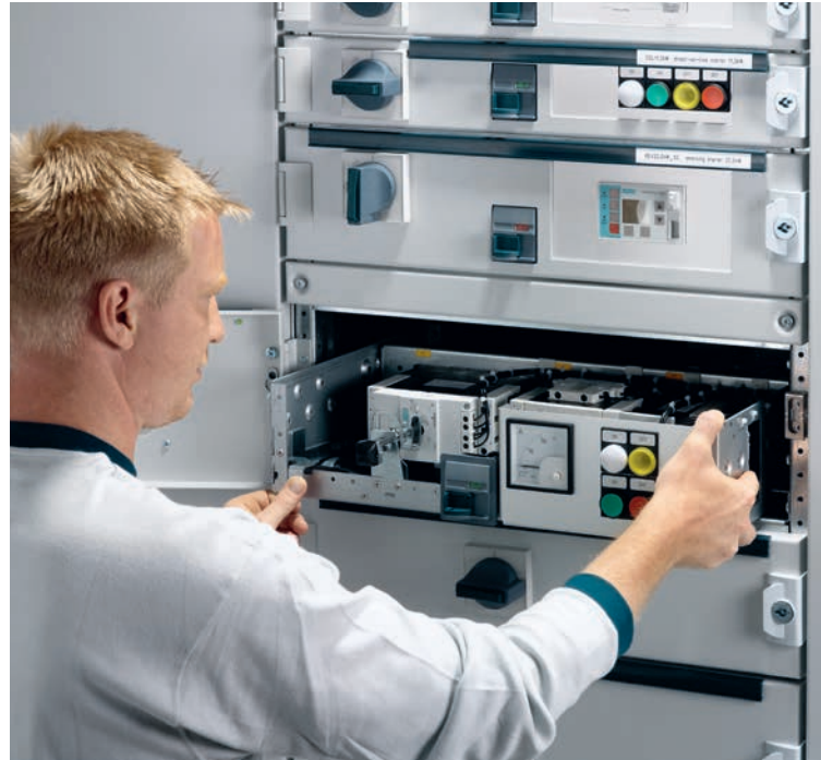
The mechanical coding of the withdrawable unit prevents any confusion of withdrawable units of the same size.
